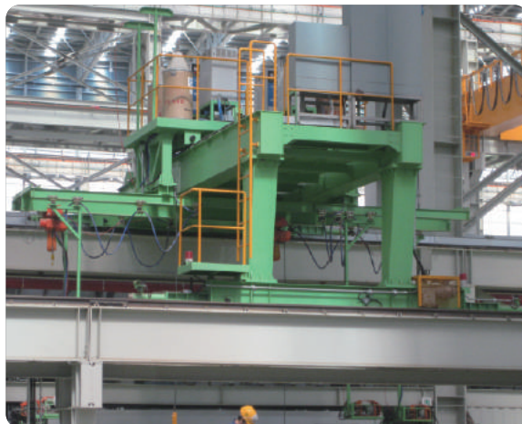
UTILITY WELDING MACHINE
